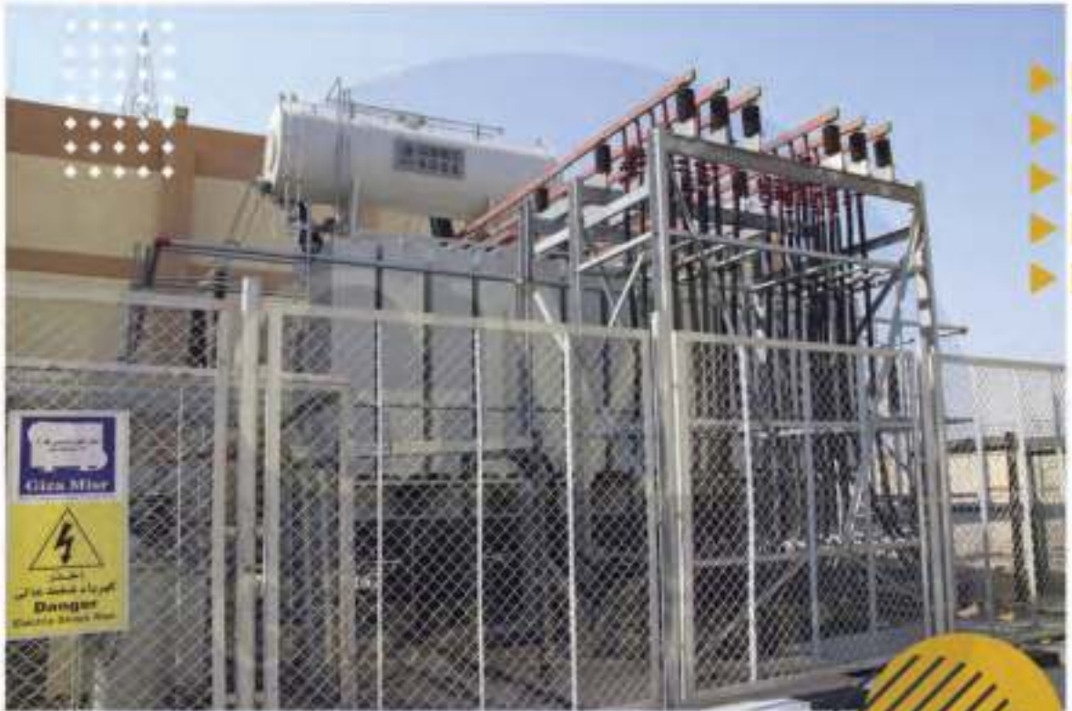
Substation West of El Shorouk 220/22/22 KV
