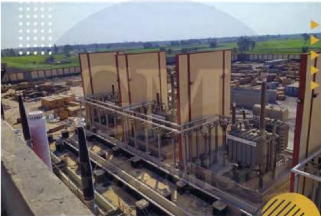
Substation Zagazig 500/220/66/11 KV
