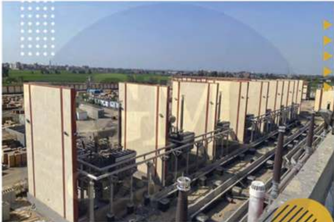
Substation Zagazig 500/220/66/11 KV
