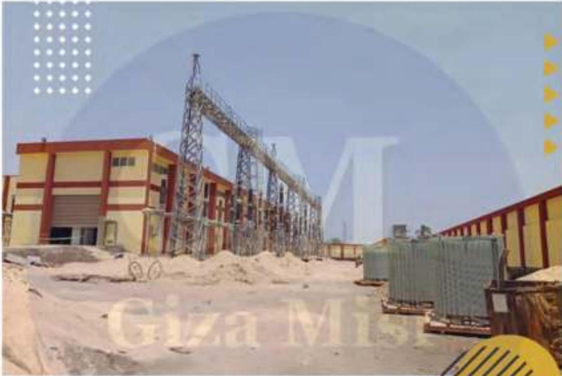
Substation Zagazig 500/220/66/11 KV
