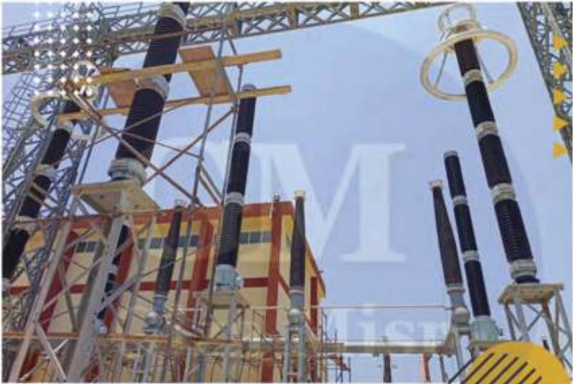
Substation Zagazig 500/220/66/11 KV
