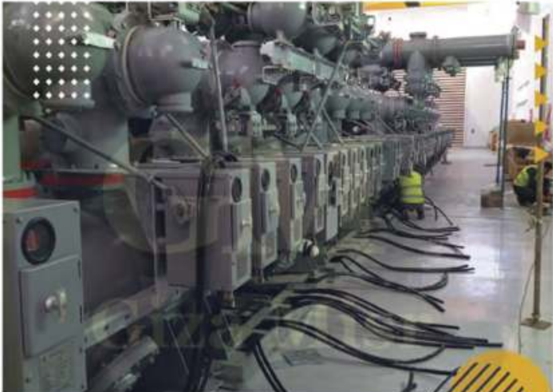
Substation Zagazig 500/220/66/11 kv
