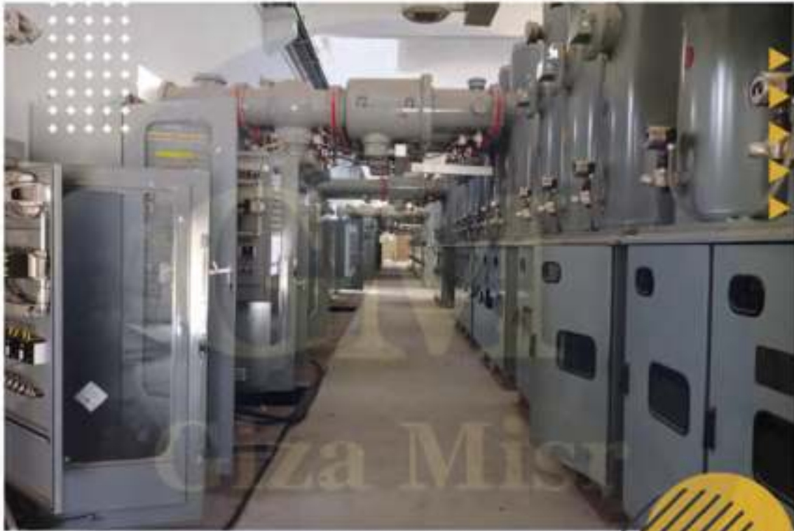
Substation Zagazig 500/220/66/11 KV
