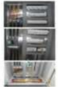
DC & AC Cabinet
