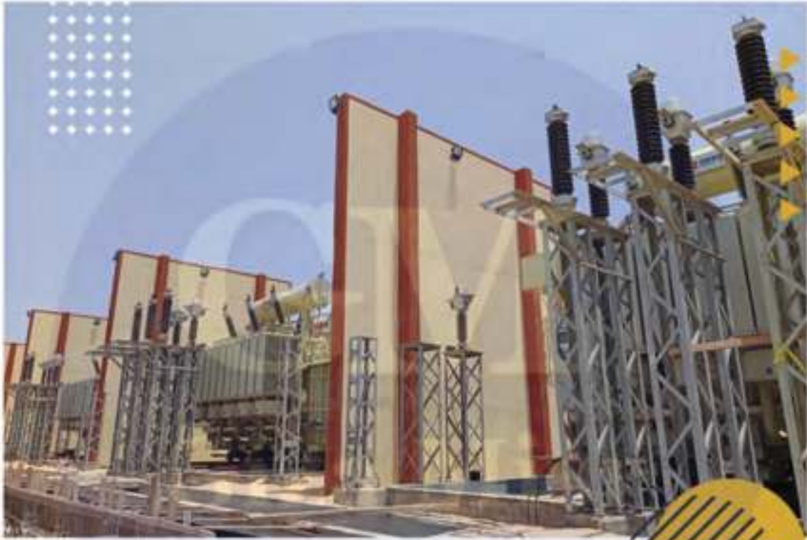
Substation Zagazig 500/220/66/11 KV
