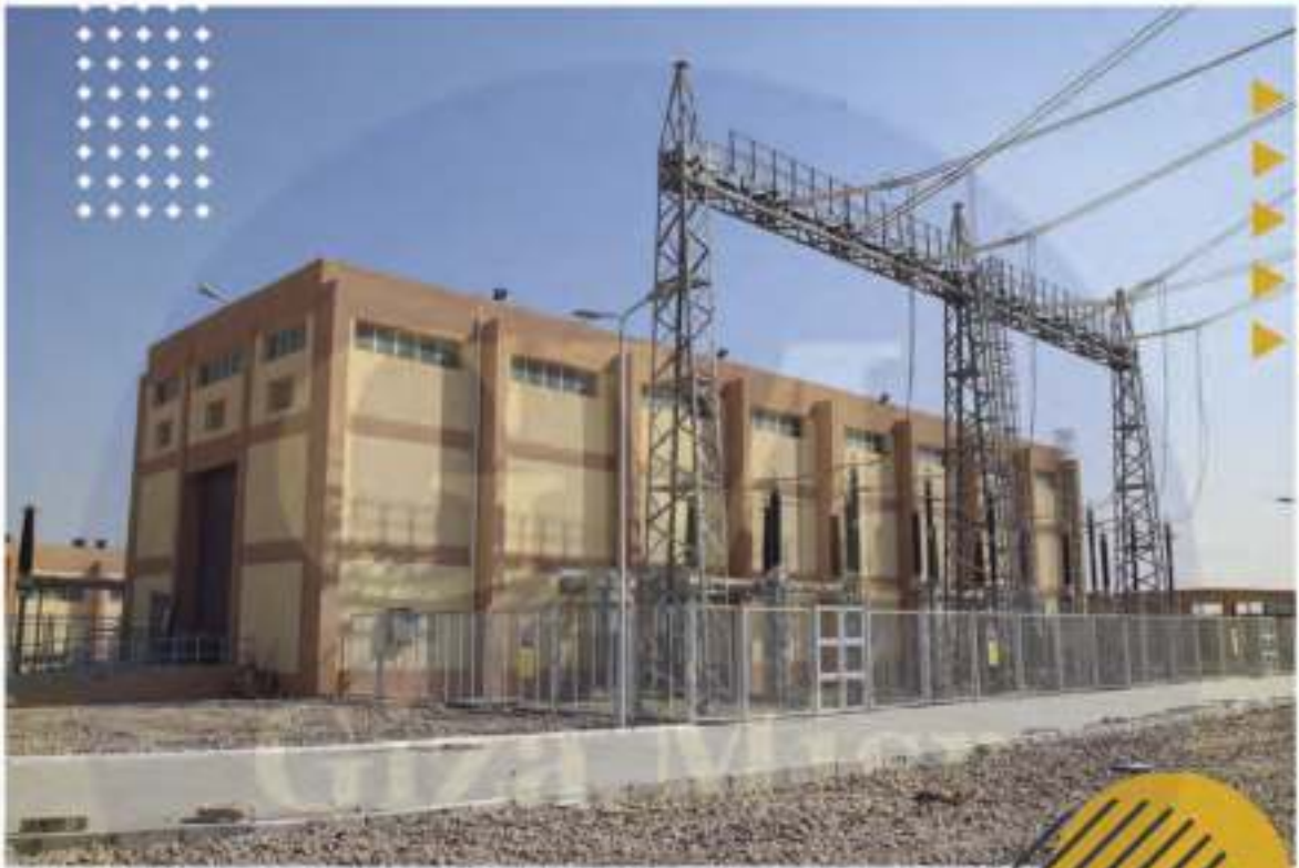
Substation West of El Shorouk 220/22/22 KV
