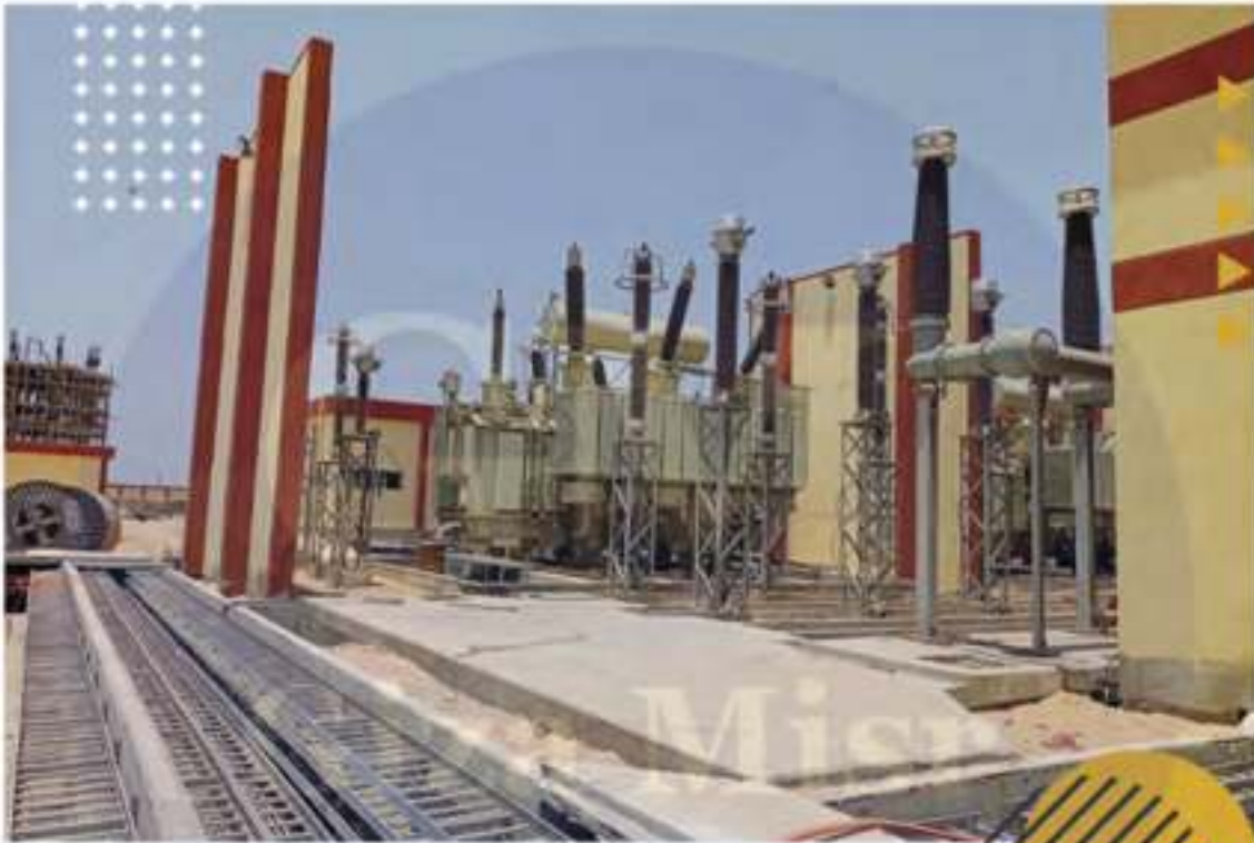
Substation Zagazig 500/220/66/11 KV
