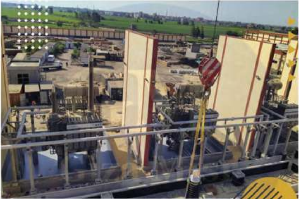
Substation Zagazig 500/220/66/11 KV
