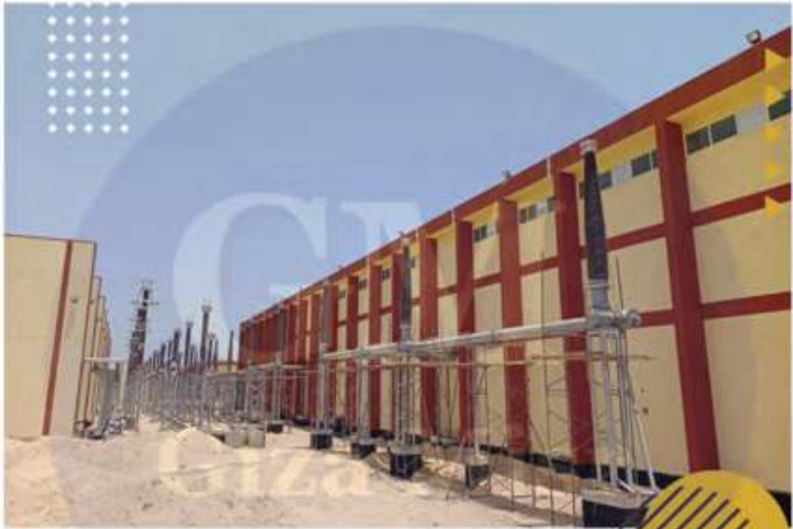
Substation Zagazig 500/220/66/11 KV
