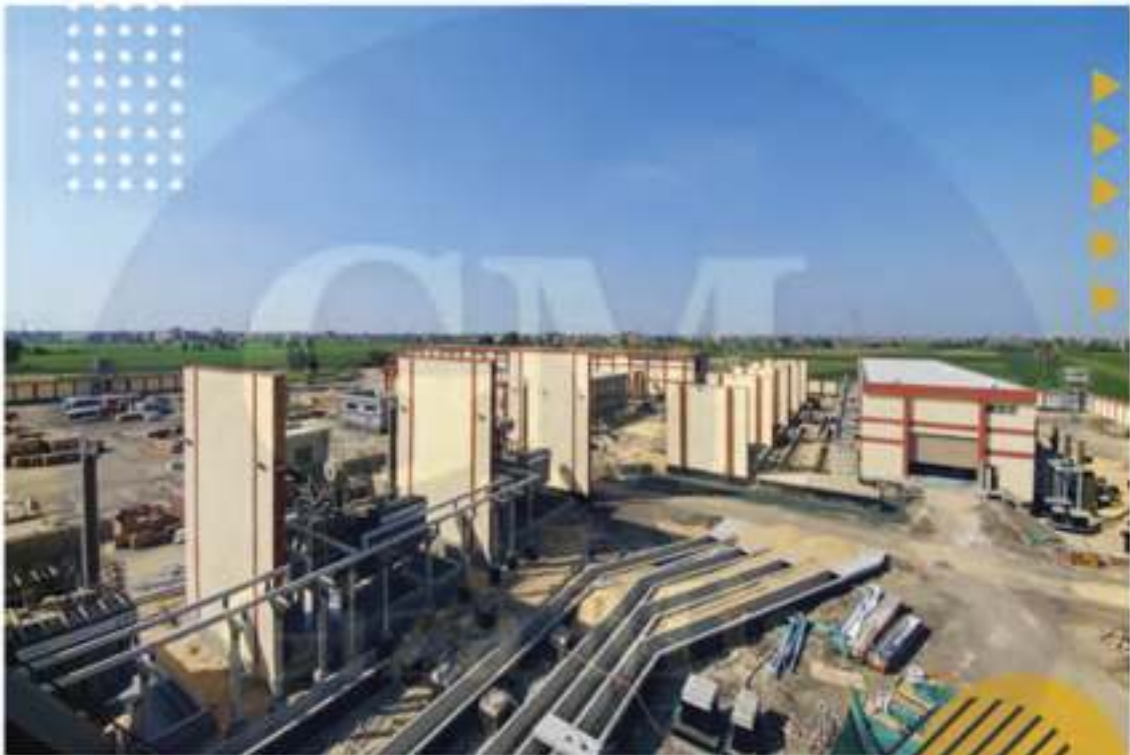
Substation Zagazig 500/220/66/11 KV
