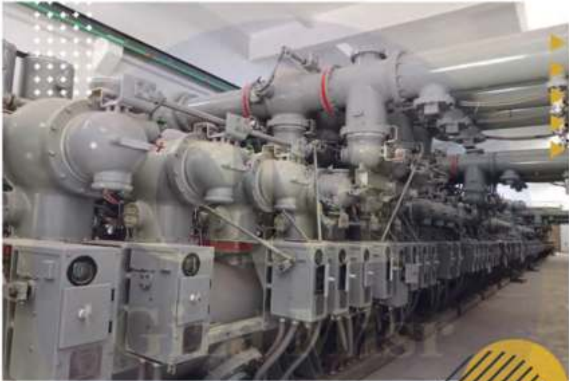
Substation Zagazig 500/220/66/11 KV
